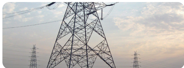
Secure reliable power sourced from CS Energy
