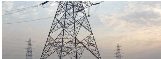
Secure reliable power sourced from CS Energy
