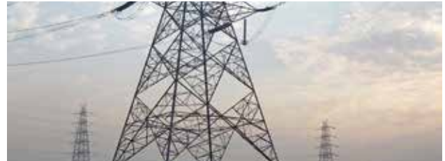
Steam is supplied to industry and power is supplied to Crescent Hadeed, Shakarganj Mills Limited and FESCO
