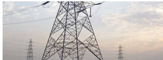
Secure reliable power sourced from CS Energy
